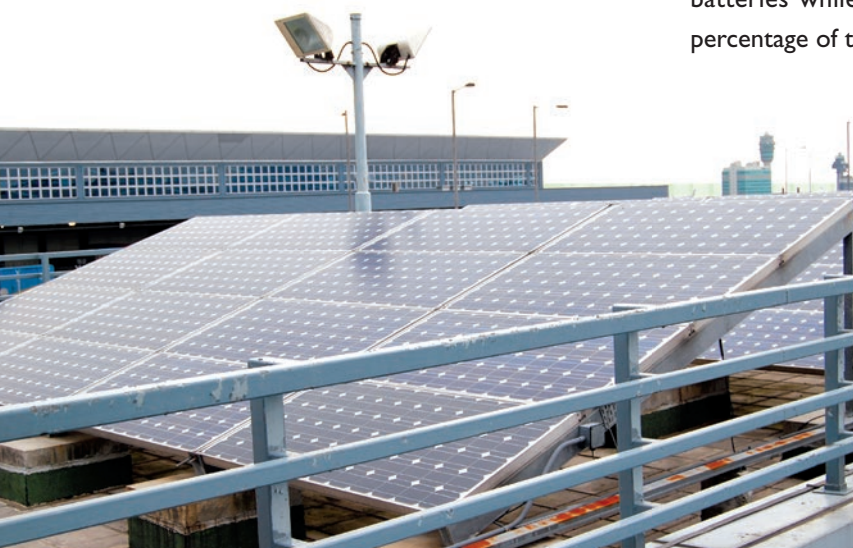
安裝在機場警署的太陽能板。 The solar panels installed in Airport Police Station.
