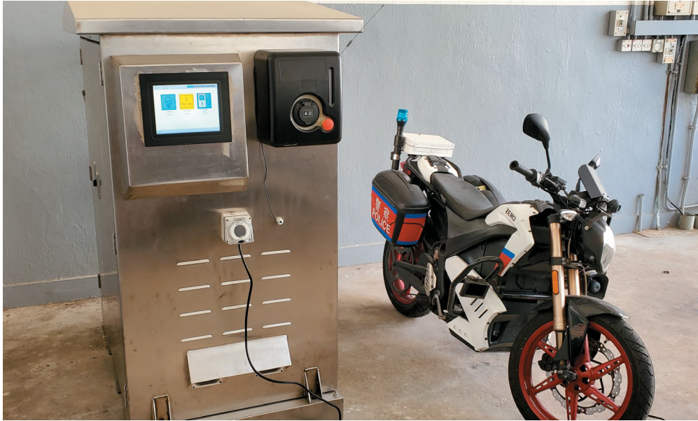
警察駕駛及交通訓練中心設有電池儲能電動車充電站。 The battery storage electric vehicle station in the Police Driving and Traffic Training Centre.
