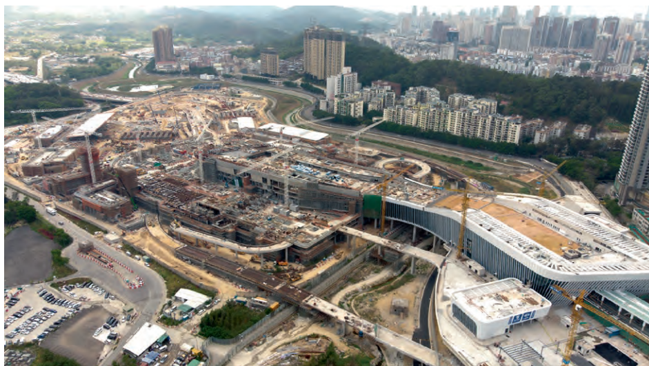
新莲塘／香园围口岸建筑工程进行中。 Construction of the Liantang/Heung Yuen Wai Control Point is in progress.
