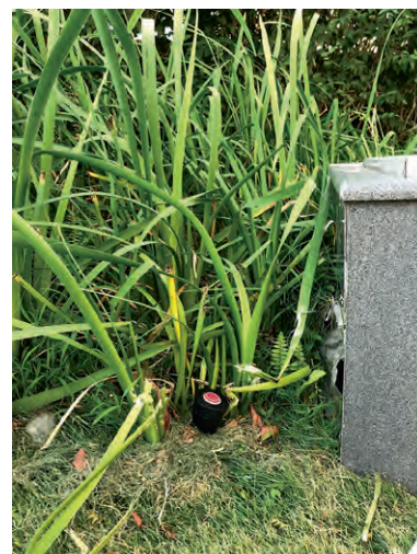
油麻地警署设有雨水循环系统。 Yau Ma Tei Police Station has installed a rainwater recycling system.
